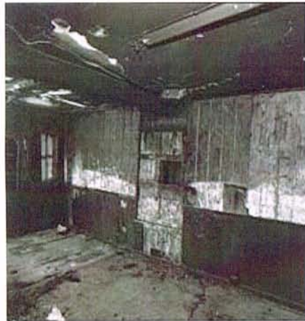
After the fire – panelling emerging from behind later boarding.
